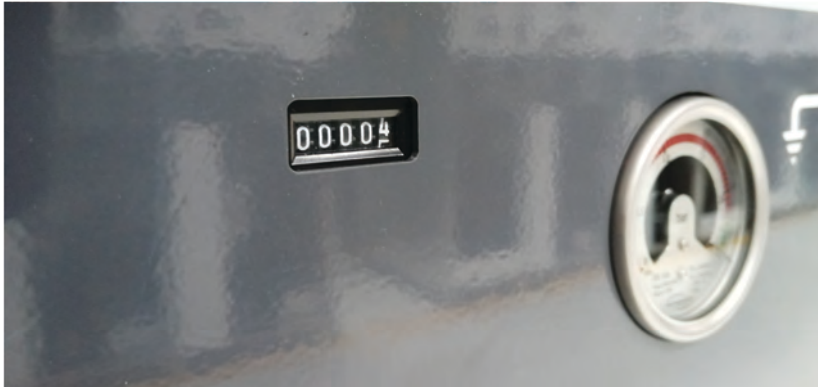
BREAK SWITCH, LOAD BREAK SWITCH ON-OFF METER APPLICATION
