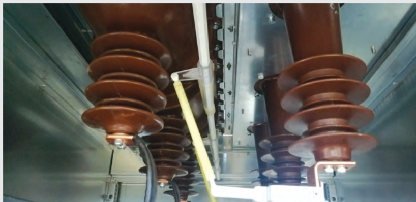
FUSE BLOWN SET
